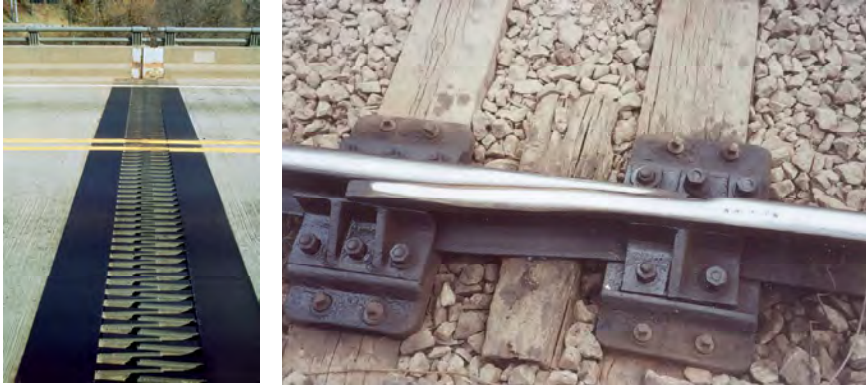
An open expansion joint on a bridge Railway line
